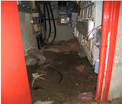
Figure 1 - Water Ingress to the Metering Installation rendering it unsafe to access the Metering Equipment
